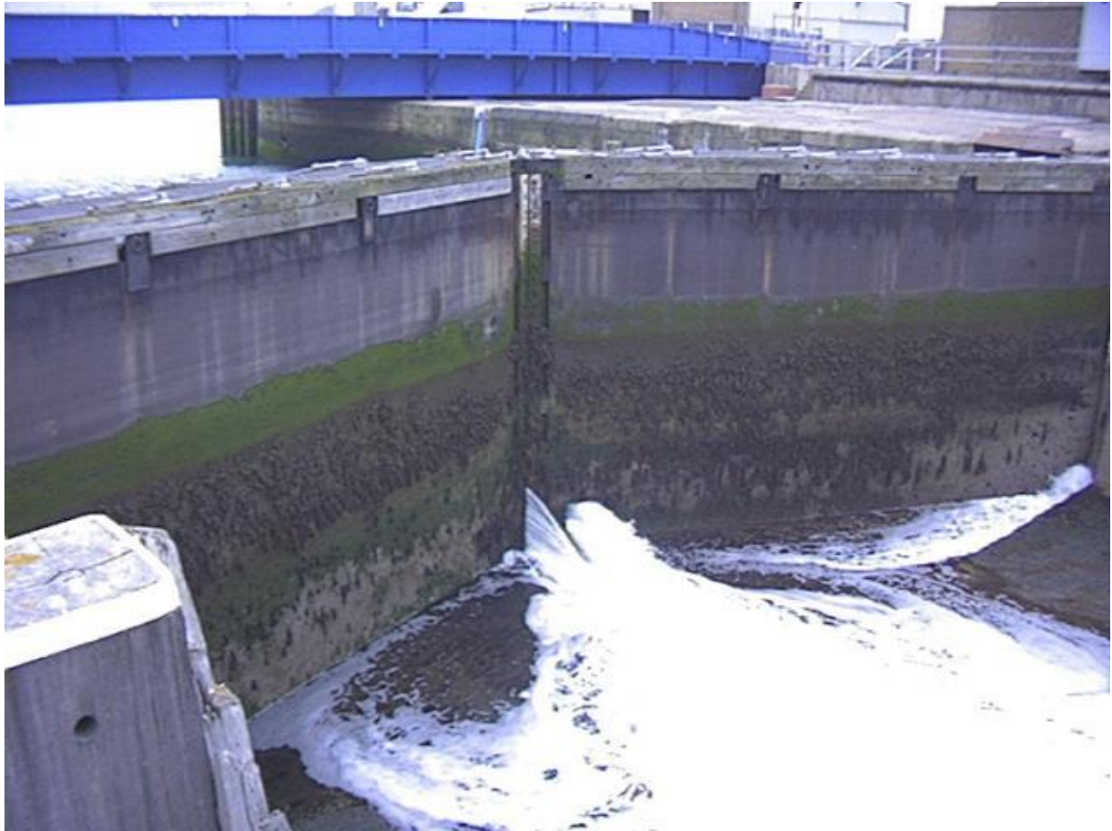
Plate 17: The dock gates at a low tide, exposing the leaking seal, looking north-east, 10/12/11, DHB.
