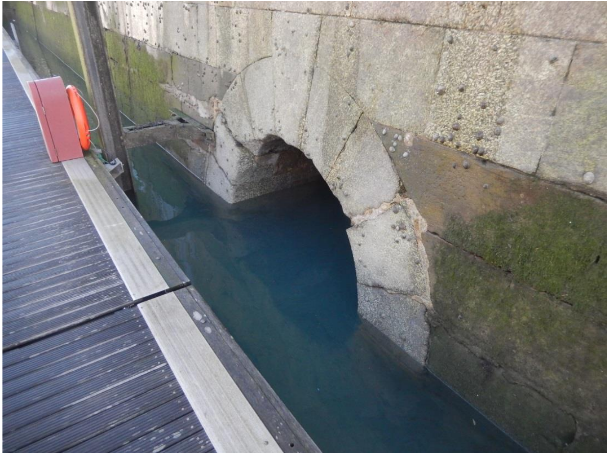
Plate 30: The culvert connected to Sluice C, present on The Crosswall, 2016, looking north-east, DHB.
