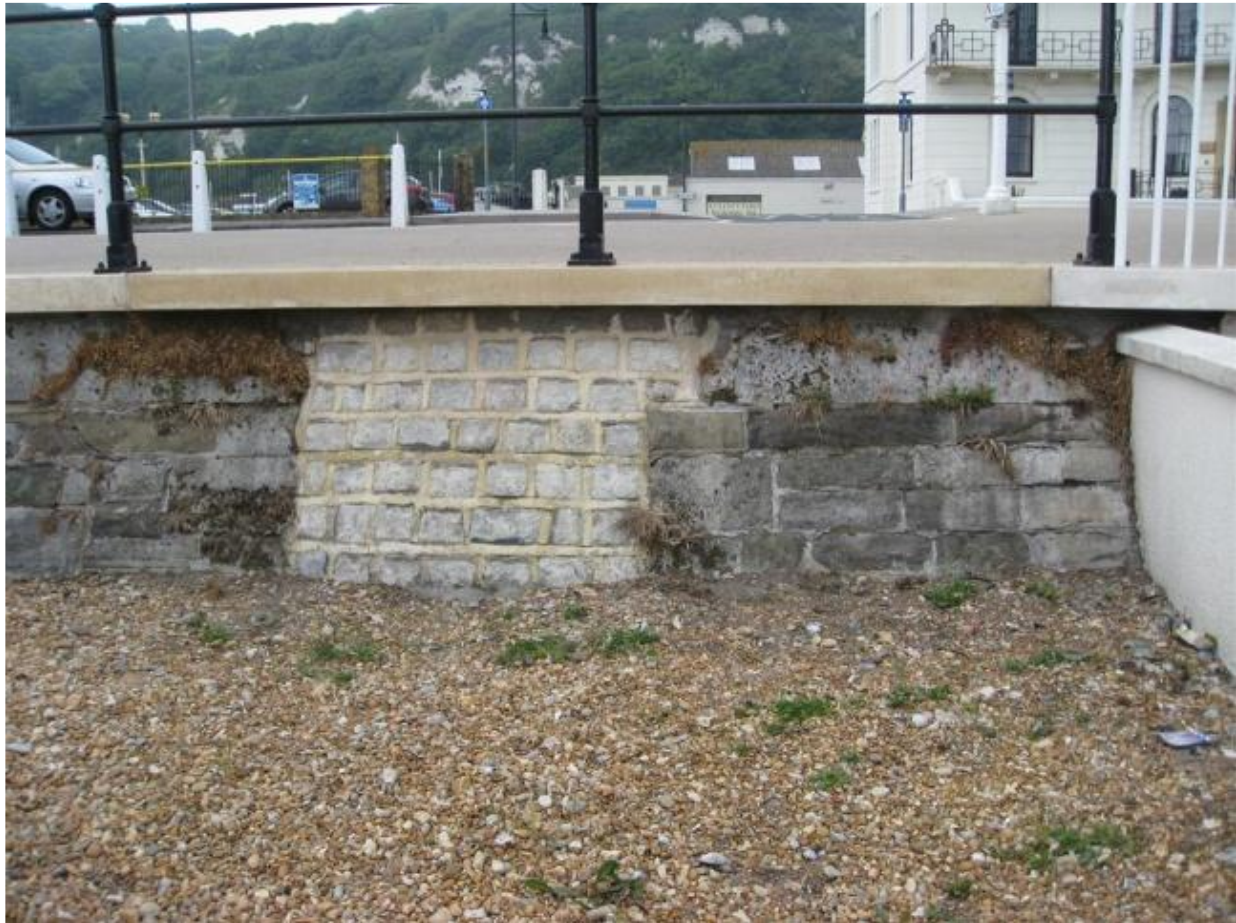
Plate 64: A section of patched sea wall showing a clear change in material, outside of Harbour House, 2013, Atkins 2014, 31.
