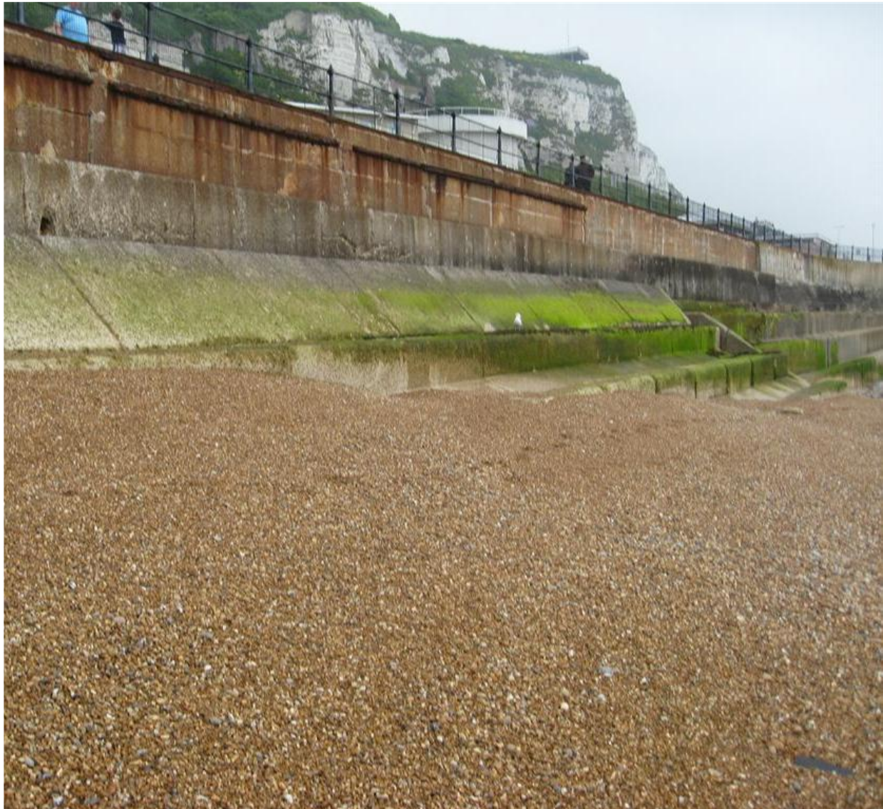
Plate 54: Marine Growth along the concrete additions to the sea wall, 2013, looking North, Atkins 2014, 19.
