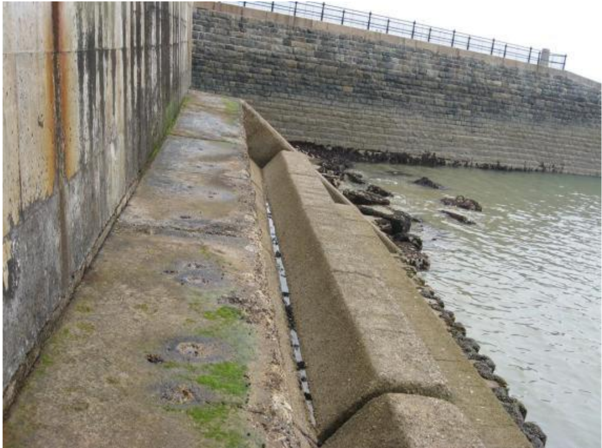
Plate 53: Concrete spalling with a masonry base, could have been installed as a tank or sea defence, 2013, looking North, Atkins 2014, 16.
