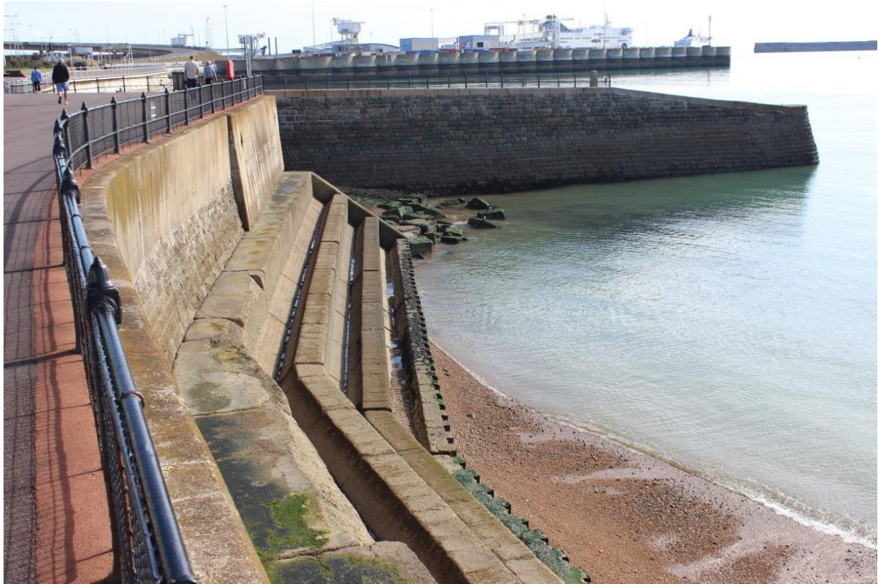
Plate 46: Old defences next to a concrete groyne- date installed unknown, 23/09/2016, looking north-east, DHB.
