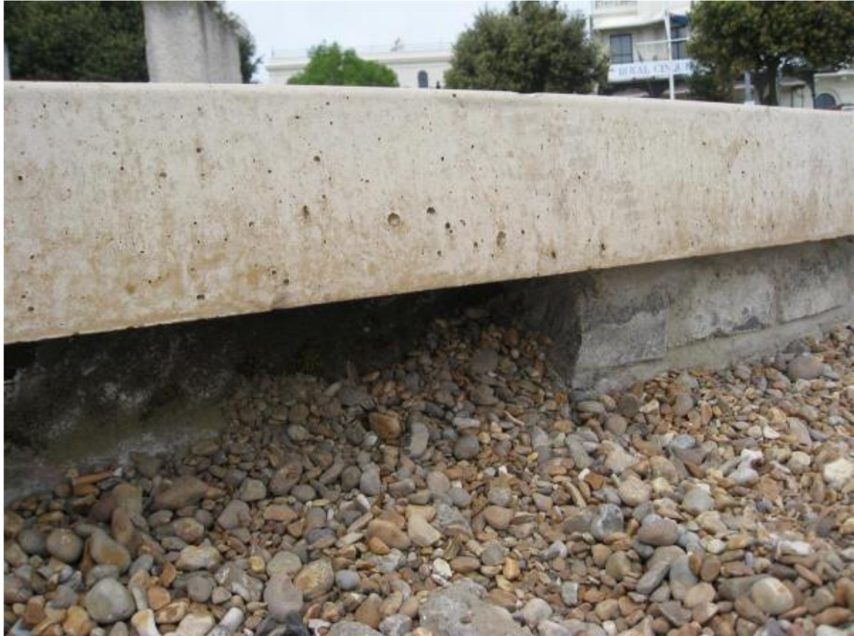
Plate 62: Undermining section further along The Promenade towards the Prince of Wales Pier, 2013, Atkins 2014, 29.
