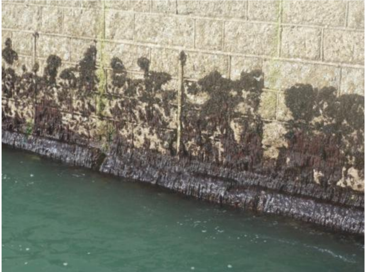
Plate 34: Low water at time of recording shows a step at the base of the pier, plans show that this form is present throughout the masonry section of the entire pier, Atkins 2014B: 35.
