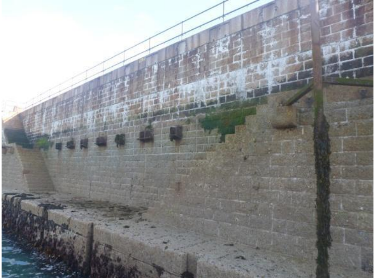
Plate 31: Two stairways which have been chained off leading down to a no longer used stage landing, Atkins 2014B: 30.
